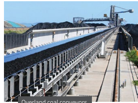
Overland coal conveyors
